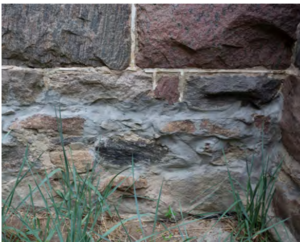
84. Evidence of later patches at cut stone base.
