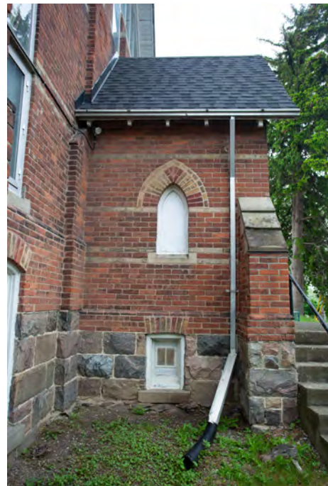
27. South facade porch, west side revealing loss of glass during 1973 fire.
