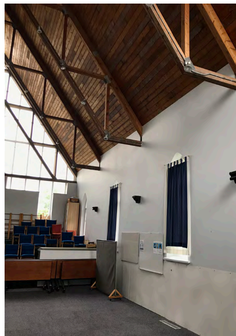
73. Interior of Dunbarton Fairport Church, view to the south, showing charred remains of corbels and beams.
