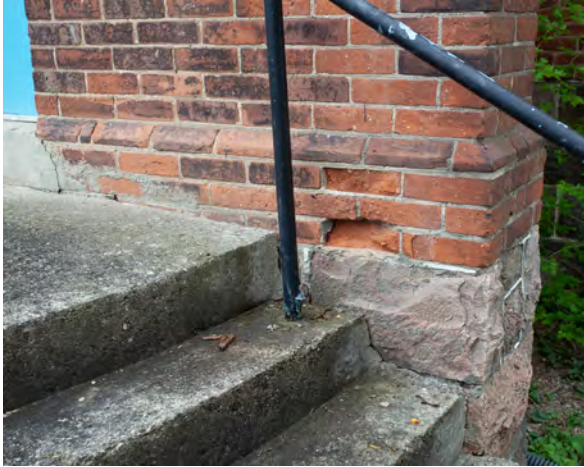
88. Spalled bricks, and separation of concrete steps at stone base, south elevation of chapel building.
