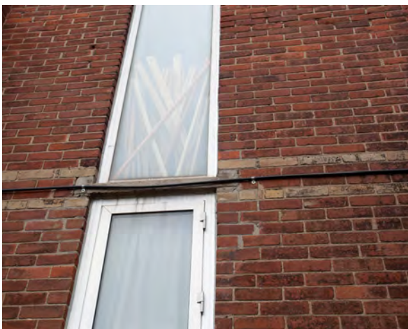
90. Curtain wall assembly and metal casement window at south elevation, chapel building.
