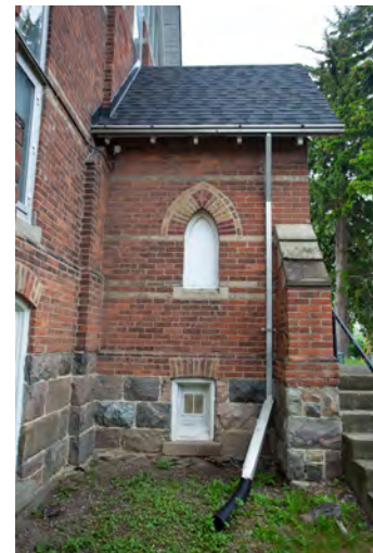
12. South Porch, West View, revealing lost stained glass during the fire of 1973. Also note the decorative dichromatic brickwork.
