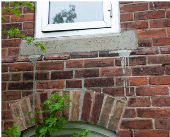
87. Later concrete sills at replacement windows, and later repointing with cementitious mortar.
