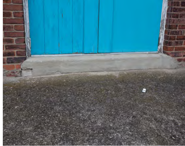
86. Chipped edge at concrete sill of entrance door, south elevation of chapel building.
