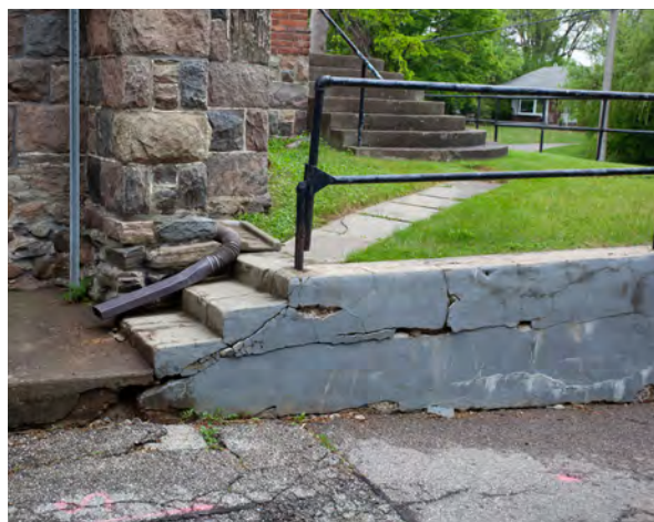
85. Damaged retaining wall at southwest corner, and exposed rubble stone foundation wall.
