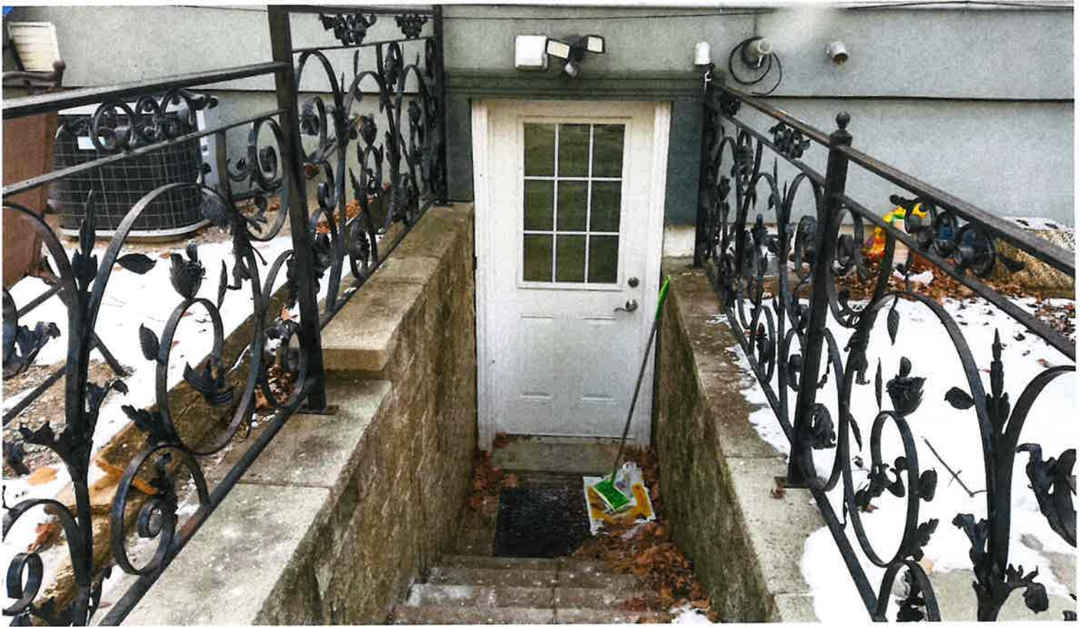
General view of the entrance to the basement at 1884 Liverpool Road at the subject site (looking South)
