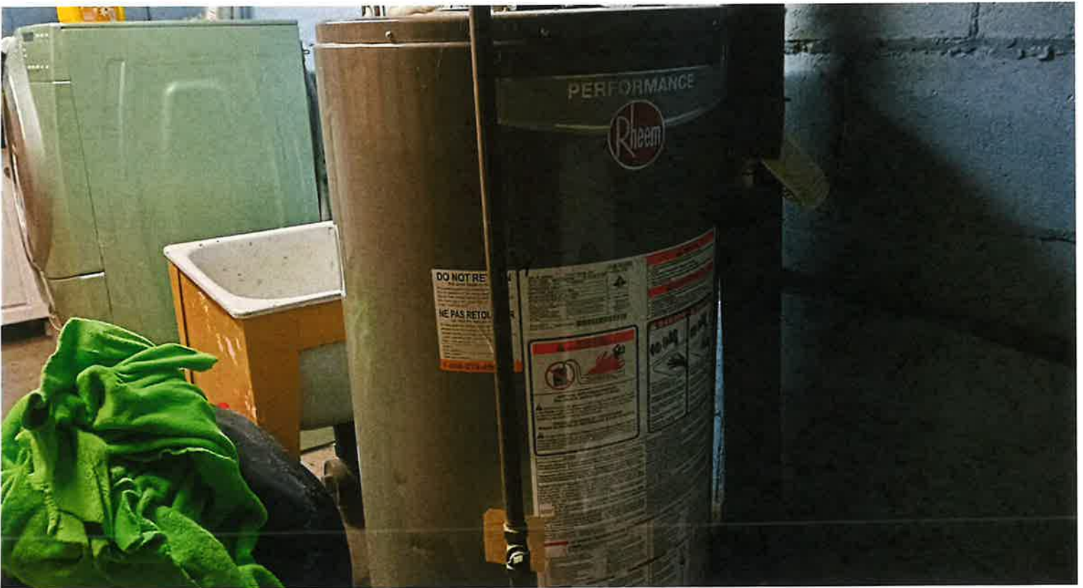
General view of the water heater in the basement at 1885 Glendale Drive (looking west)
